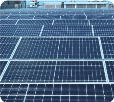
Solar Panels with Capacity of 1.7MW
