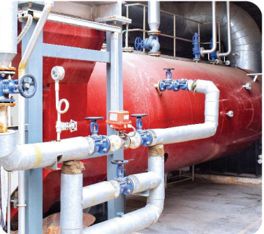
Waste Heat Recovery Boilers
